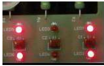
Fig. 2-12 LED indication when V phase is open.
